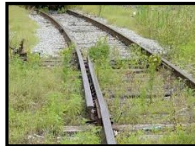
Split Point Derail
