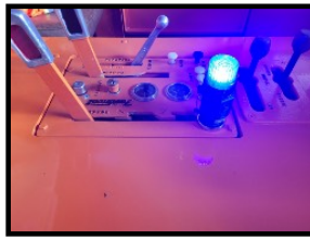
Blue Light on Control Panel
