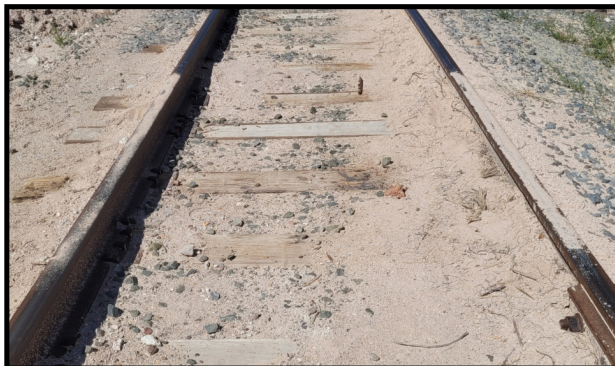
Sand On Top of Rail
