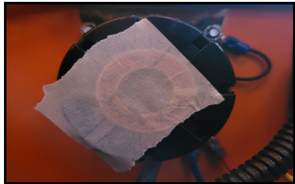
“Taped Over Turntable Alarm”
