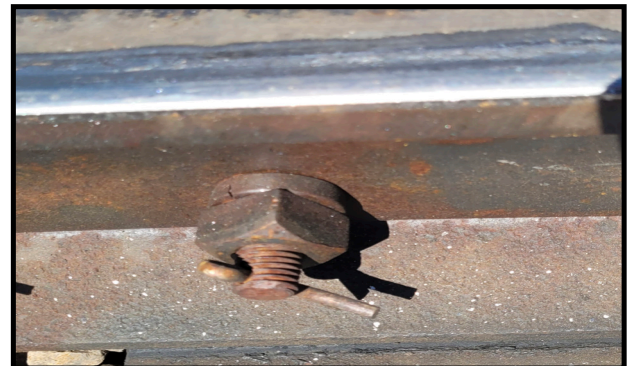
Metal Grindings at Base of Rail
