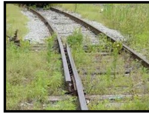
Split Point Derail
